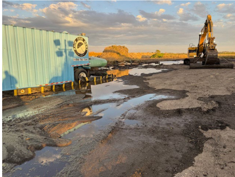
Facing north at Milepost 31.2, north of County Highway 9/135th Street, spilled hydrostatic pressure test water within the topsoiled ROW, did not leave silt fenced perimeter, October 5, 2025
