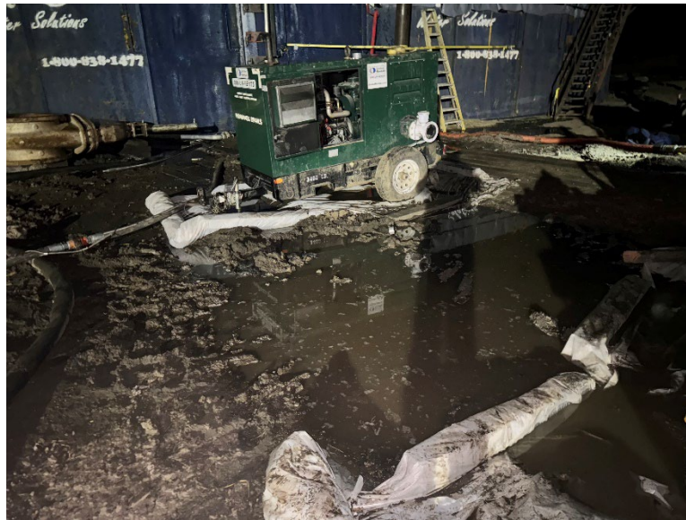
Facing northwest at MP 34.2, north of 165th Street, spilled hydrostatic pressure test water within the topsoiled ROW, did not leave silt fenced perimeter, during draining of the pipe October 7, 2025
