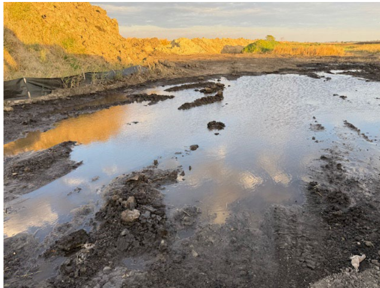
Facing north at Milepost 31.2, north of County Highway 9/135th Street, closer view of spilled hydrostatic pressure test water within the topsoiled ROW, recently excavated and stabilized subsoil piles in background, October 5, 2025
