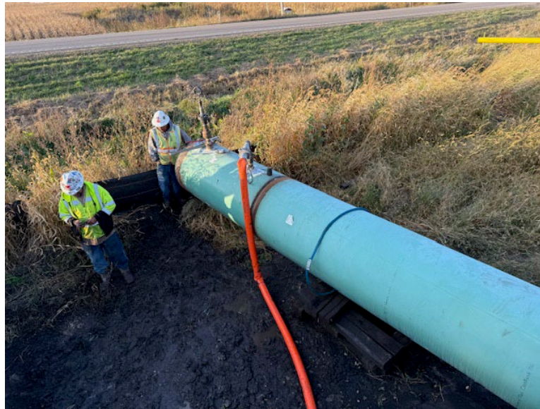
Facing south at Milepost 31.2, north of County Highway 9/135th Street, origin point of the hose that came out of the tank, during filling of the pipe October 5, 2025
