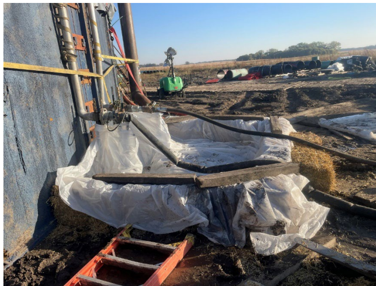
Facing northeast near milepost 34.2, secondary containment build under fill pipes and hose connections
